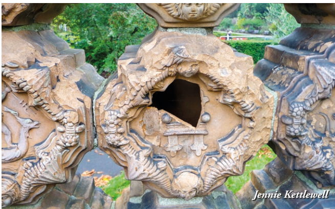
Damaged terra cotta brick
